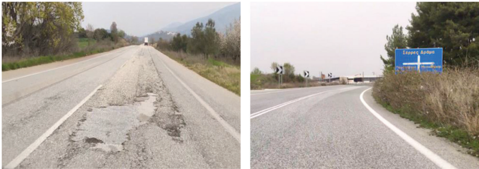
Figure 6: Lack of maintenance of pavement and signing.
