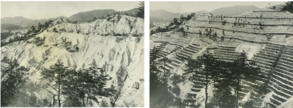
Figure 1: Bare land in Japan before (left) and after (right) greening work. In the greening work, saplings are planted along the contour lines of the terrace where the slopes have been cut out [9].
