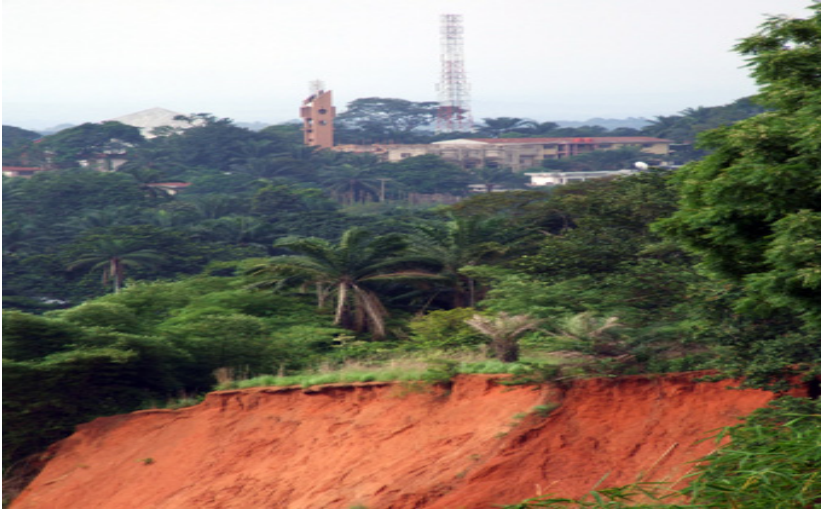
Figure 2: Collapse of river bank as a result of gully erosion in Southeastern Nigeria.
