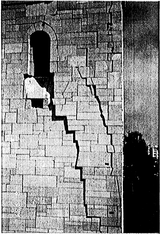
Figure 4: Severe cracking and displacement at tower
