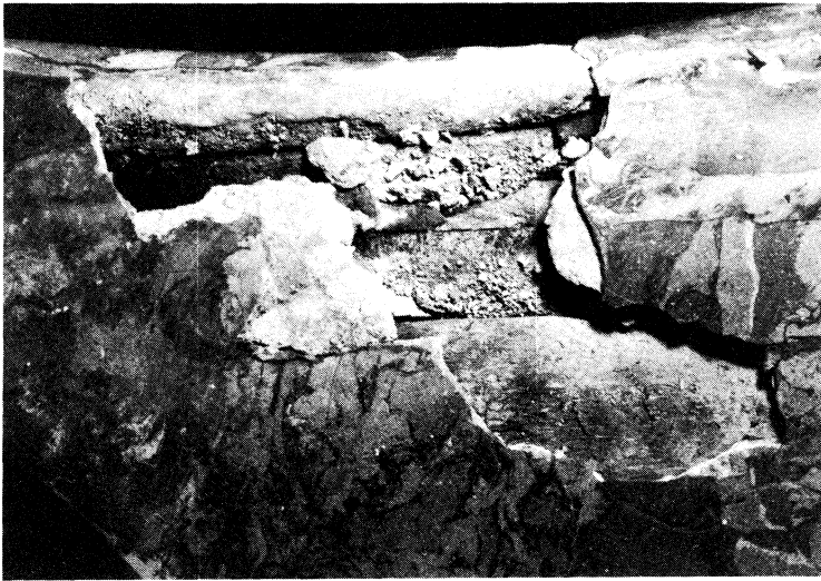
Figure 2: Church of Lichtenfels, missing and loose parts in the stucco marble layer and the plaster
