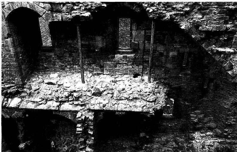
Figure 2: New posts supporting massive overhangs. tube supports constructed from cold formed stainless steel. These have been installed to support major
