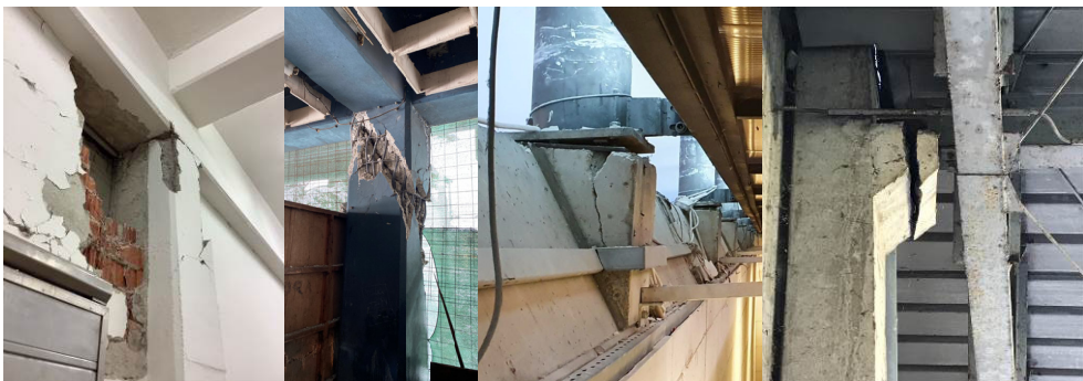
Figure 3: Damage to RC structures. (Source: [10] and authors.)
