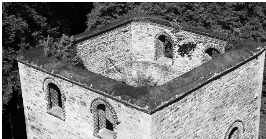
Figure 4: Missing roof and vegetation of Brockhauser Tiefbau (picture by Hensing/Knappenverein Schlängel u. Eisen).
