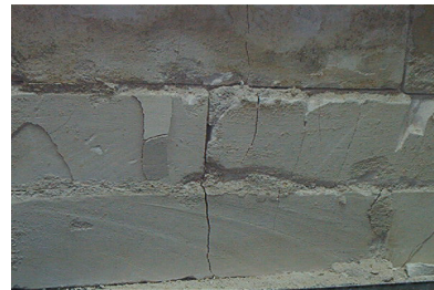
stone tensile cracking and crushing
