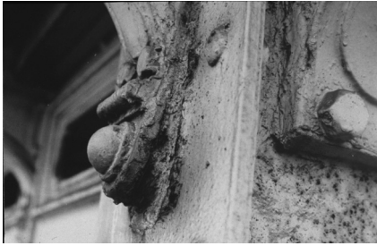
Figure 1: Platform roof HS Station Den Haag. Crevice corrosion between the cast iron bracket and the wrought iron strut. The pressure of the rust has demolished the bracket.
