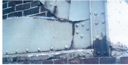
Figure 2: Engine House, Zeche Zoller II, Dortmund-Bövinghausen. Severe corrosion has occurred on the facade between the masonry and the framework.
