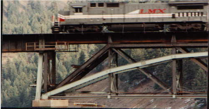
Figure 7: Montanal Rail Link Bridge rehabilitated for the AREA Cooper E80 (1.472 million pounds live loading).
