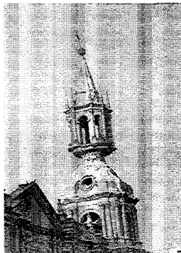
Figure 4: Right Tower Damage
