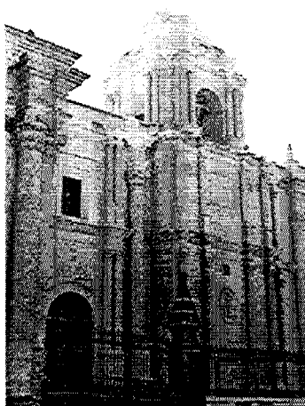
Figure 3: Left Tower Damage
