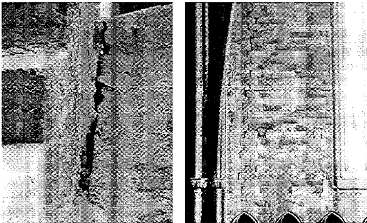
Fig. 8. Cracks developed in the junction between arch and vault (Mallorca Cathedral, left.) and in a construction joint (Girona Cathedral, right)
