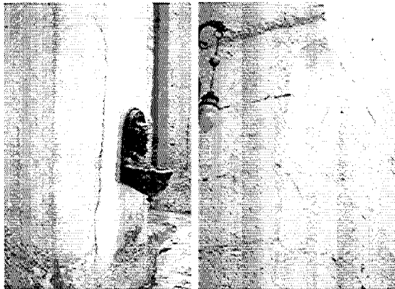
Figure 16: Siracuse Cathedral. Crack pattern of a pillar
