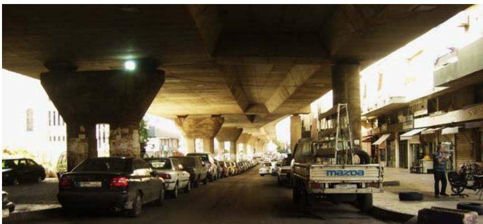
Figure 6: A Place under Yerevan Bridge. Most of sectors are built by single loaded columns. (Photo credit to Aram Papazian.)
