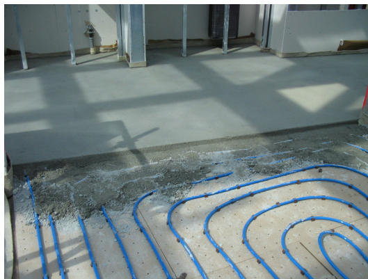
Figure 6: Radiant panels for heating system.
