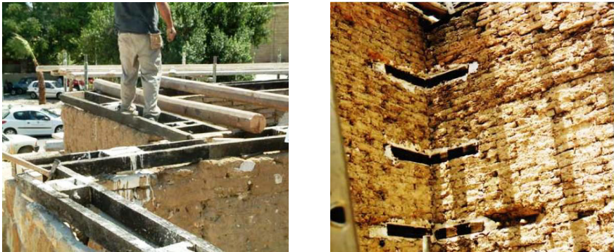
Figure 6: Installation of a wooden ring beam on the upper part of an adobe structure (left) and of timber beams at the corner of adobe walls (right).
