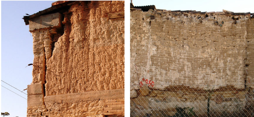
Figure 4: Building exhibiting various forms of structural damage such as the deterioration of its upper part, the disintegration of adobe and the formation of detachment cracks (left). Slumping of adobe wall that has been caused by the deterioration of its base (right).
