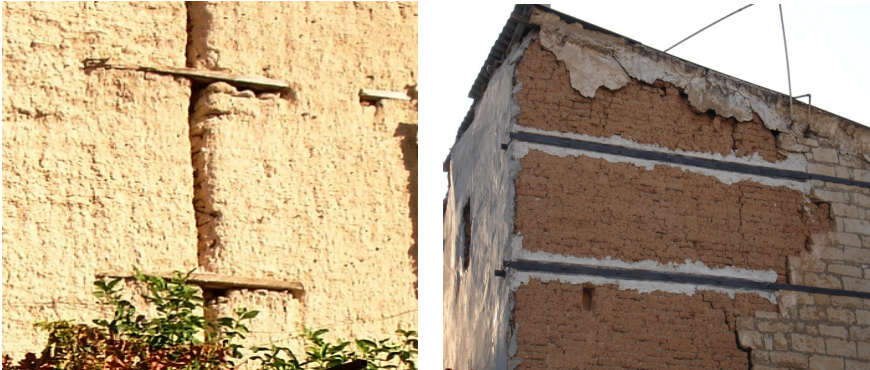
Figure 5: Installation of timber beams for the treatment of a vertical discontinuity (left). Steel straps that have been installed in an adobe structure to repair cracking (right).
