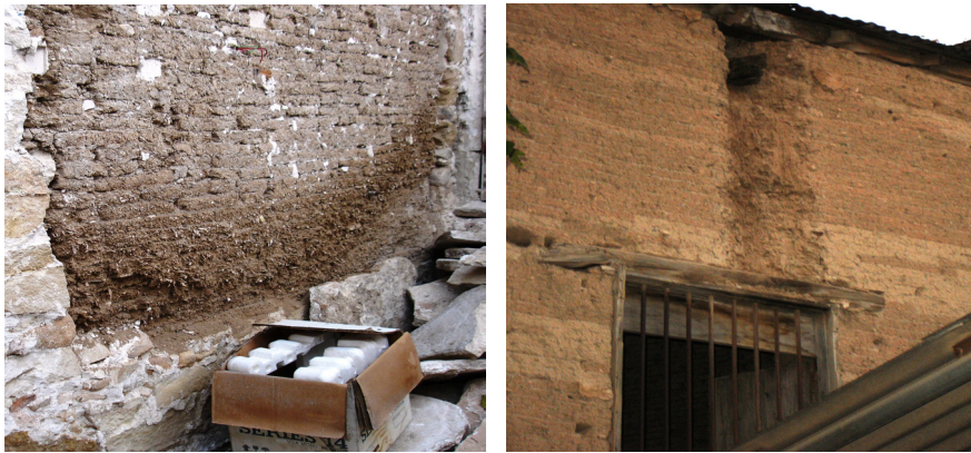
Figure 2: Deterioration at the base of an adobe wall (left) and characteristic fissure on the upper part of an adobe wall caused by the action of rainwater (right).
