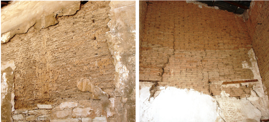
Figure 3: Disintegration of adobe and loss of the protective coating as a result of trapped moisture and water washing down the surface of the wall (left). Various vertical and diagonal cracks in the body of an adobe wall (right).
