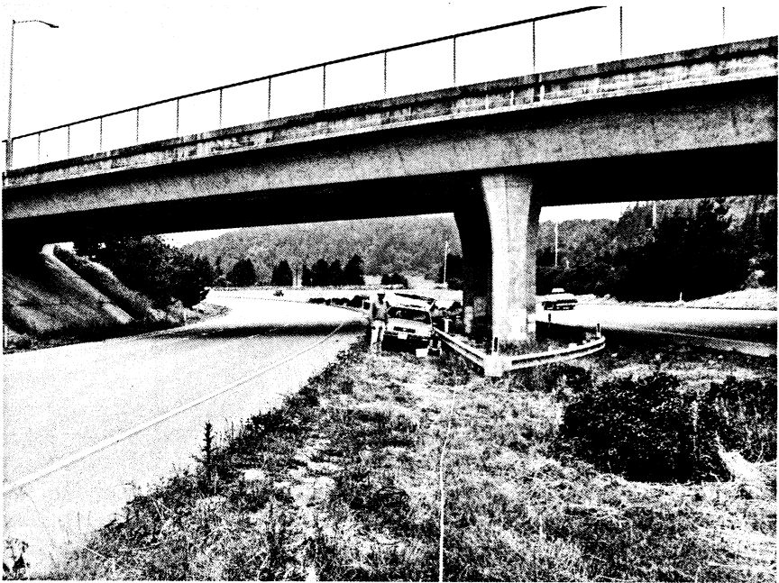
Figure 2: The Painter Street Bridge in Rio Dell, CA, and location of the Petrolia Earthquakes of April 1992.
