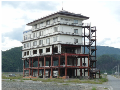
(c) Damaged hotel in Taro City
