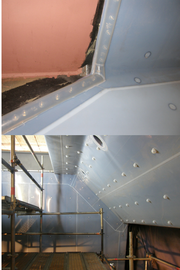
Figure 6: Examples for PFA linings fabricated on a high technical level. Transition zone (upper) and lining of a housing with two diverging fix point application methods (lower). Courtesy Plasticon Europe, D-Dinslaken.
