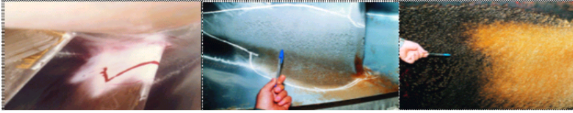
Figure 2: Cracks in the runner, cavitation damage on the blades surface, and cavitations on the draft tube surface.
