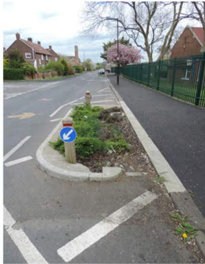
Figure 2: Embleton Road site-visit, May 2017. (Source: Bristol City Council 2015 [32].)
