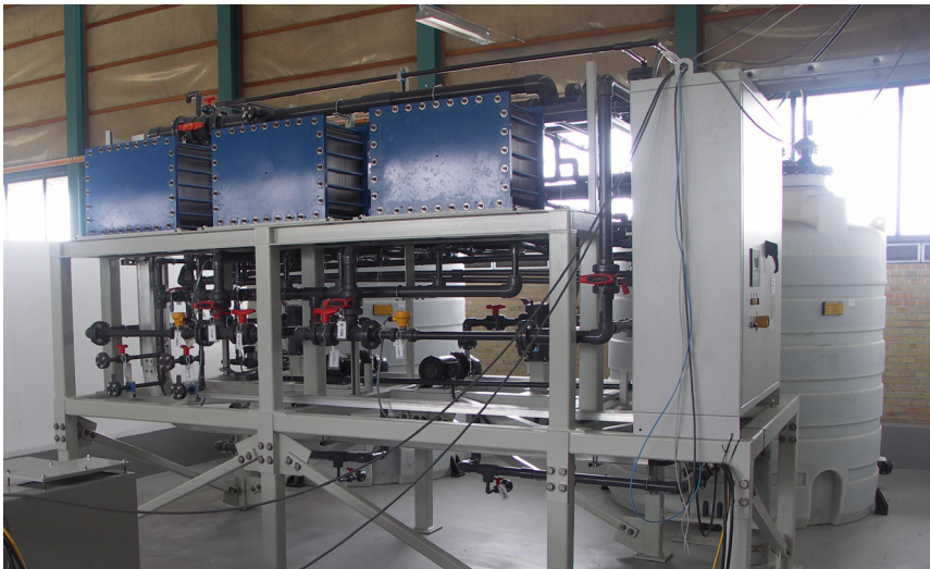
Figure 2: Photo of the vanadium battery installation at SYSLAB. The three blue units in front are the cell stacks, each containing 40 cells. Behind the cell stacks and the pump/pipe system, the two 6500 liter electrolyte tanks are situated. The box to the right is the control unit.
