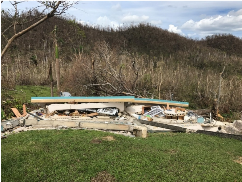
Figure 7: In some parts of the island, winds from Hurricane María destroyed concrete structures entirely.
