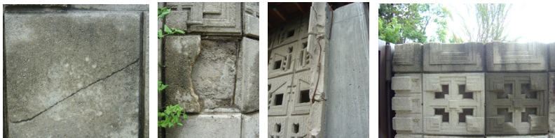
Figure 5: Typical damage, photos – Angela Paola Vargas – 2004.
