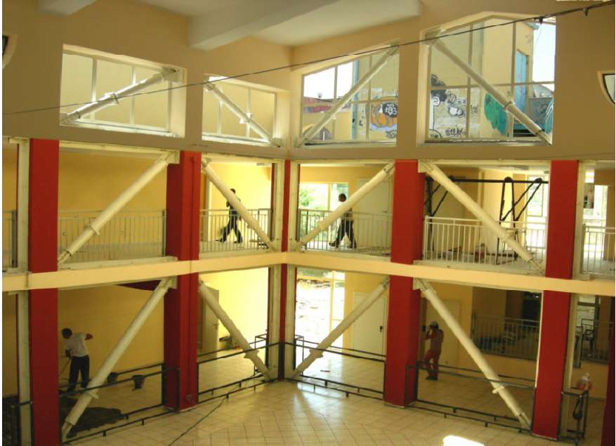
Figure 5: Buckling-restrained axial dampers installed in the School “Cappuccini” in Ramacca, Italy (courtesy of Prof. Fabio Neri).
