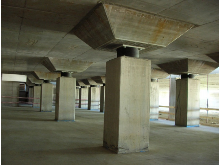
Figure 3: Elastomeric isolators installed in the Ospedale del Mare, Naples, Italy.
