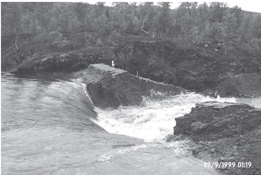
Figure 22: View of breach formation.
