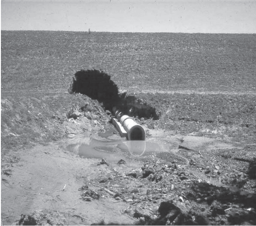
Figure 18: Failure by piping along conduits (after [16]).
