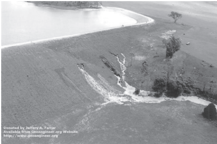
Figure 17: Failure by piping, Tunbridge dam, Tasmania, Australia (available from Geoengineer.org website).
