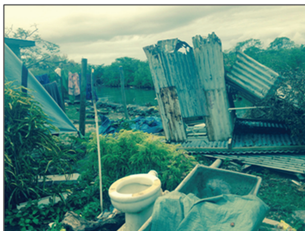
Figure 2: The remains of a family home and bathroom on Qoma Island. Image courtesy of Rowan Gard.
