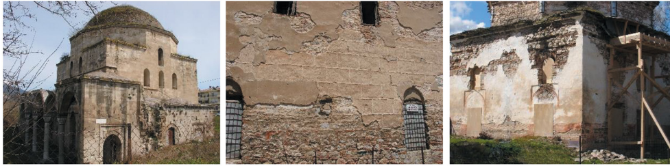
Figure 9: (a) View of Mehmet Bey mosque, (b) loss of plaster at Koursoum mosque and (c) loss of plaster and the presence of colour at the mosque of Exochi.
