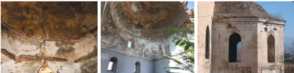
Figure 7: Cracking in the three monuments: (a) Orta mosque, (b) Ahmet Bey mosque and (c) Mehmet Bey mosque.
