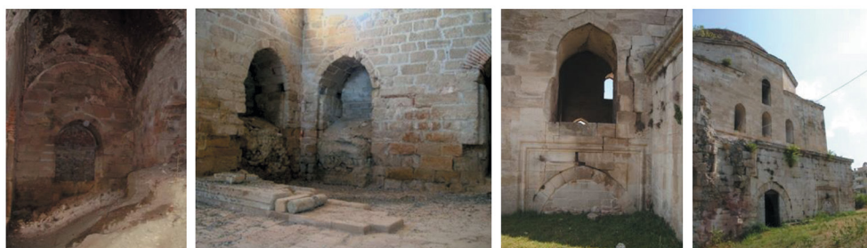
Figure 12: Views of Mehmet Bey mosque where the interior and exterior space is full of debris.
