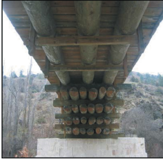
Figure 26: View from the cantilever beams and main beams of the historical Bayramören Bridge in Çankırı (after restoration) [16].
