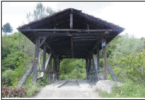
Figure 22: The upper structure of historical Dörtocak Bridge in Kastamonu (Photo credit: S. Yılmaz, June 2016).
