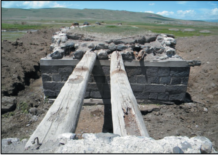
Figure 16: The view from the deck of the bridge of the historical Pular Bridge in Erzurum [12].
