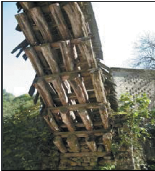
Figure 21: The view from cantilever beams of the historical Buzlupınar Bridge in Rize [10].
