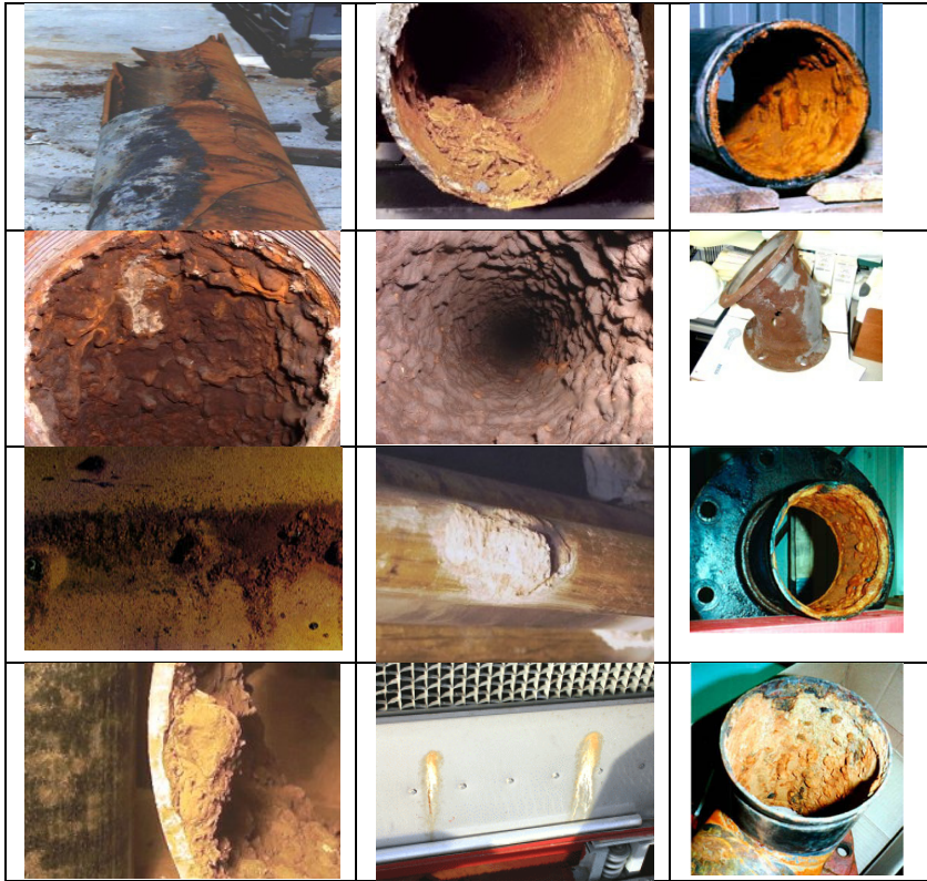
Figure 2: Different types of corrosion of metallic water pipelines.
