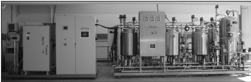
Figure 2: Ozone CIP pilot plant.
