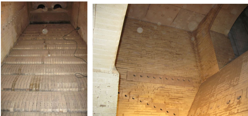
Figure 2: Grate in primary combustion chamber and secondary and tertiary air inlets.
