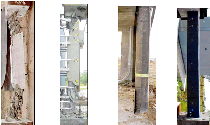
Figure 7: From left to right: RC column (field test), RC column (blast simulator test), CFRP wrapped column (field test), CFRP wrapped RC column (blast simulator test).
