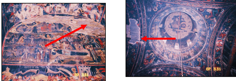
Figure 9: Damage of the internal transverse wall and the adjacent arch.
