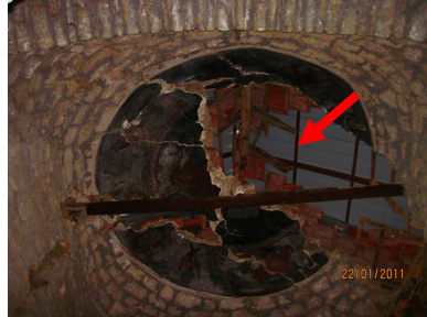
Figure 3: Damage to the South-East corner.
