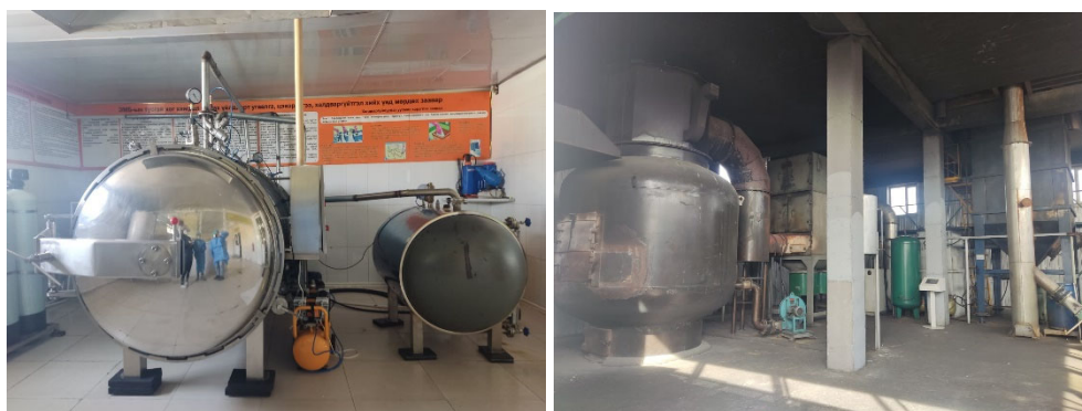
Figure 2: EM's autoclave (left) and incinerator (right).
