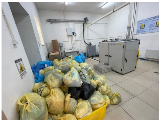
Figure 4: NW15 steriliser installed at the NCMCH.
