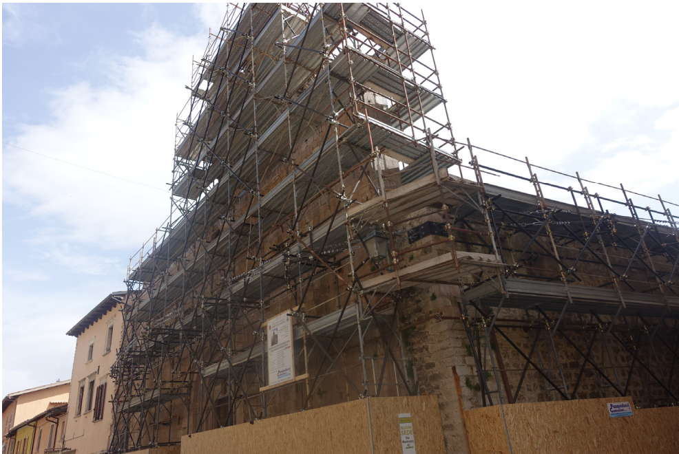
Figure 2: Leonessa – Detail of a church damaged by the seism. (Source: Author's archive.)
