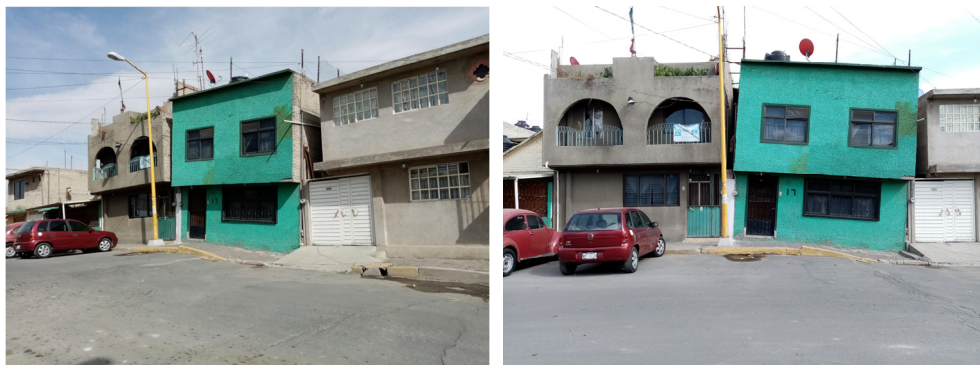
Figure 3: Affectation of soil cracking in modified housing. Loss of verticality. UH Ermita Zaragoza neighbourhood. (Source: Alonso Baca, 2021.)
