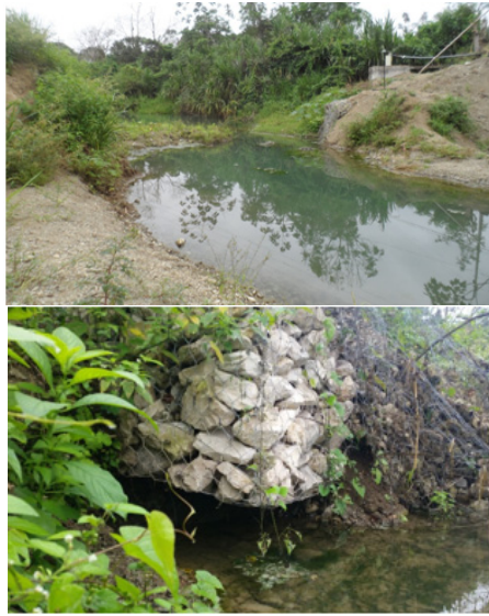
Figure 7: Tape failure during the rainy season. (Source: [15].)
