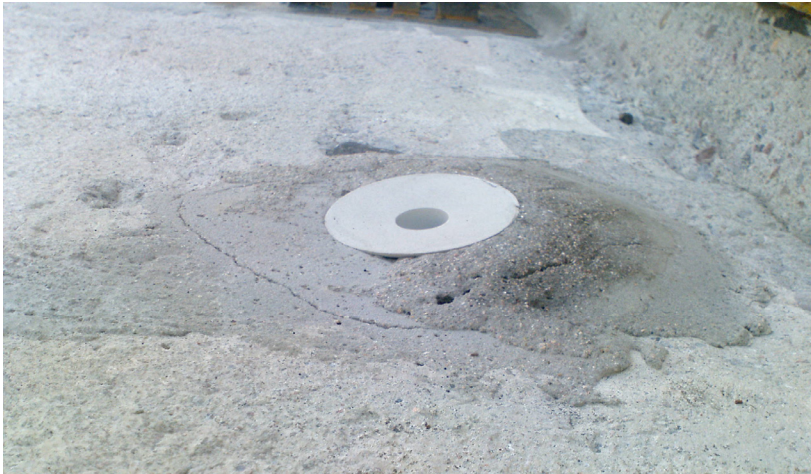
Figure 4: Concrete surface not suitable for installation of waterproofing (photo: Mikael Kinnmark, DAB Domiflex AB).
