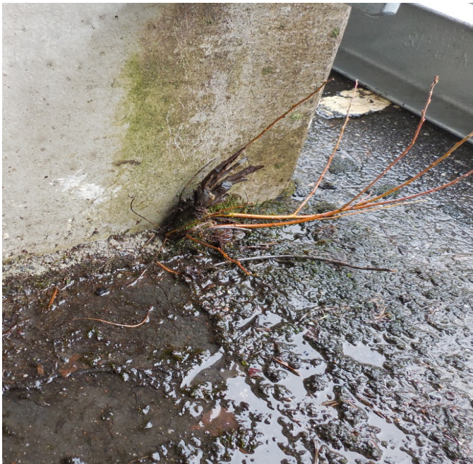
Figure 3: Concrete may need protection (photo: Dennis Lundgren, CBI).
