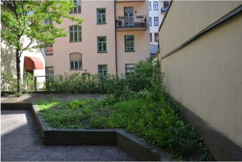
Figure 5: Green roof courtyard causing leakage in the garage below ground.
