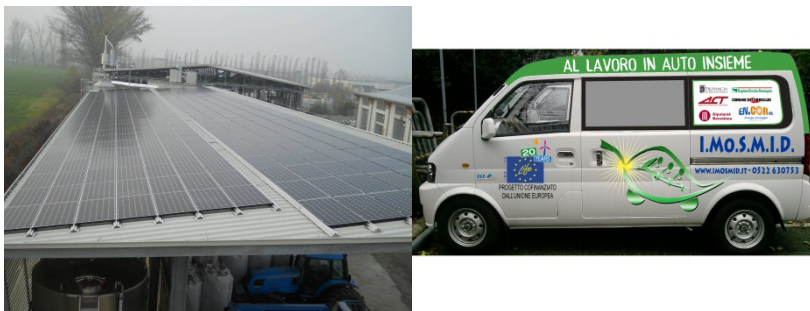
Figure 5: Photovoltaic shelters and electric vehicles used in the project.
