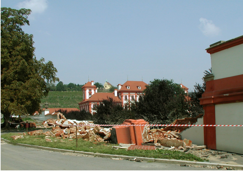
Figure 1: Failed garden wall subjected to water pressure and flow.
