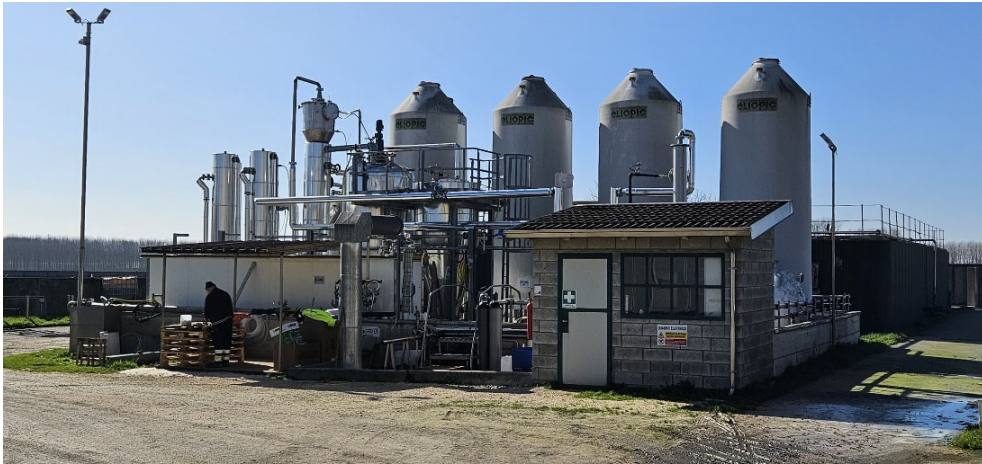
Figure 1: Ingénia technology section in the existing biogas cogeneration plant.
