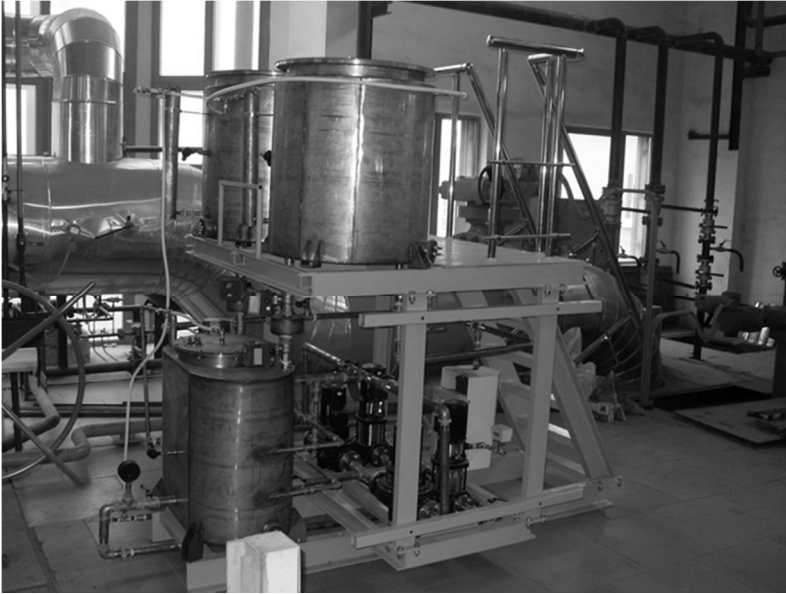
Figure 1: The stationary automated installation of SAS technology implemented in closed heating systems.
