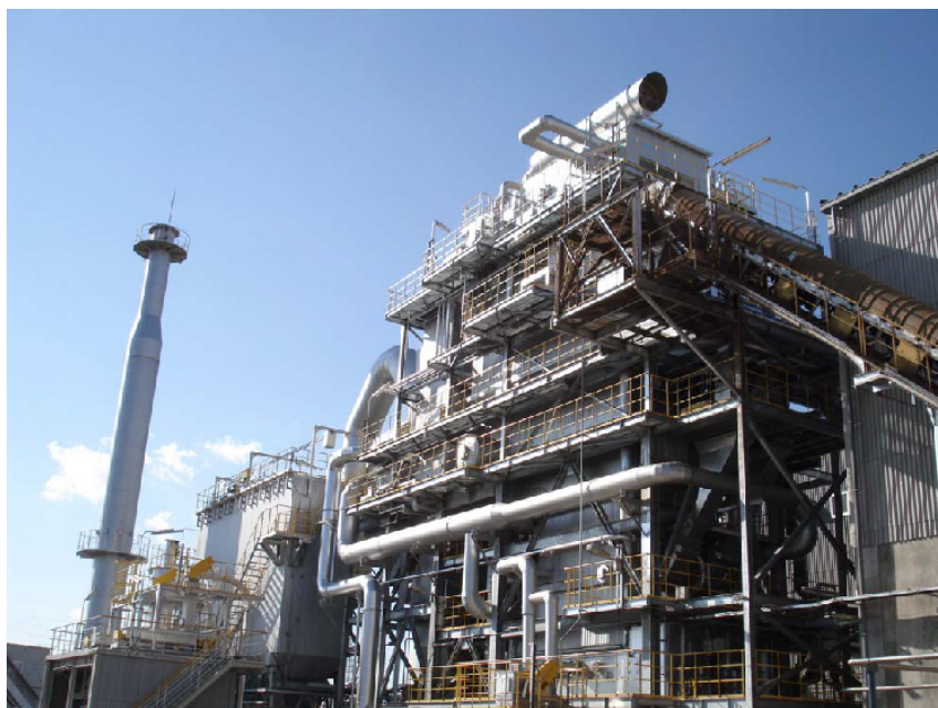
Figure 3: Woody biomass-fueled steam and generator facility commissioned into service at the DIC Kashima Plant.
