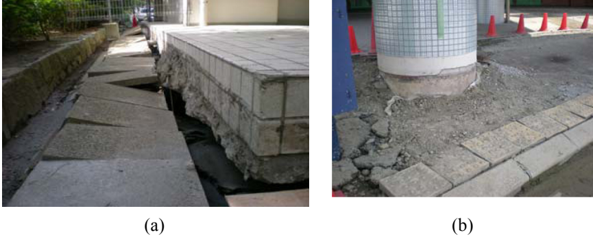
Figure 6: (a) Contact point of foundation and ground. (b) Contact point of footing and ground.
