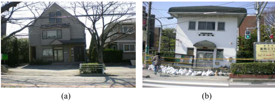
Figure 5: (a) Tilting of a small residence. (b) Tilting of a police station.
