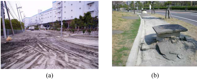
Figure 7: (a) Boiled sand on the road. (b) Lifted manhole.
