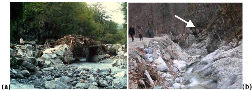
Figure 6: The bridge between reaches 9-10: (a) from downstream right after the flood; (b) from upstream two months later. Source for a: http://www.davca.si . The arrow indicates the flood marks.
