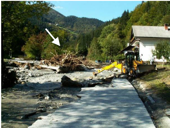
Figure 8: Channel aggradation and channel avulsion along reach 12, with a bridge clogged by LW. Source: www.davca.si .
