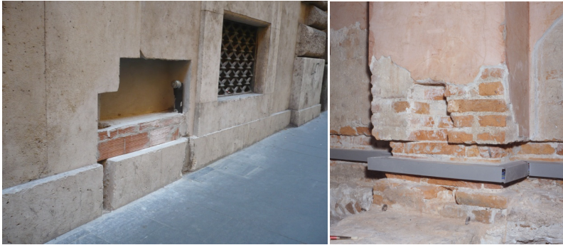
Figure 1: Niche performed on a masonry wall of a building in the historic center of Rome adjacent to a window. Cut in the walls and in pilasters of Milan's Palazzo Reale for the passage of electrical conduit.
